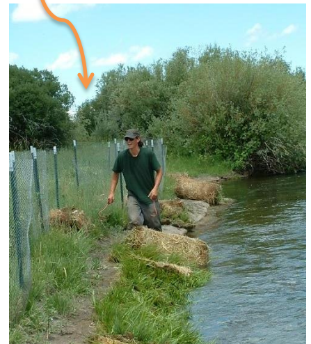
Revegetated streambanks are more stable, provide fish and wildlife habitat and capture sediment.
