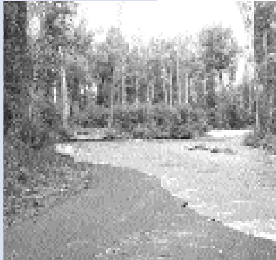
Here today ... 400' of the bike path along Teton Creek at Creekside Meadows was removed by high flows (approximately 700 cfs) in May and June.
