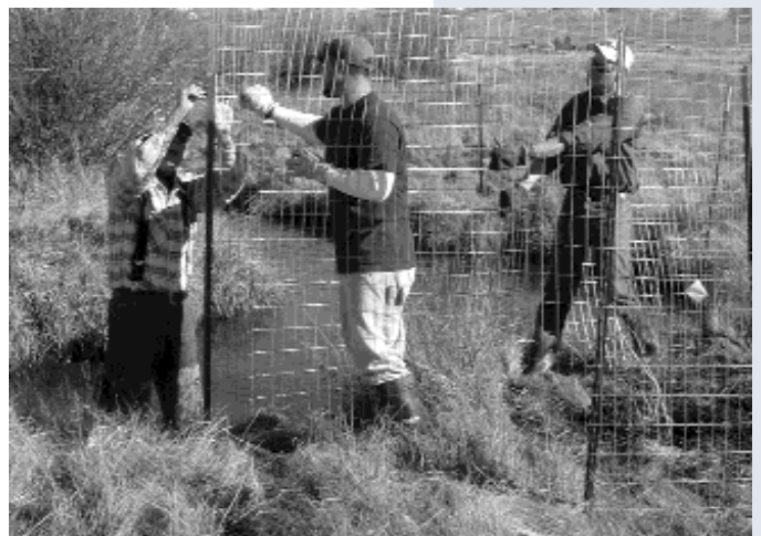
Tom Fenger, Adam Taylor, and Art Svejda install fencing to protect plants from moose and deer.
