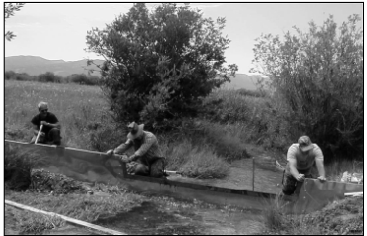
USGS Geological Survey hydrologists install a stream-flow measurement weir on Six Springs Creek.
