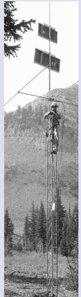
Solar panels (above) provide the electricity needed to operate the new Snotel site (below) at Grand Targhee.
