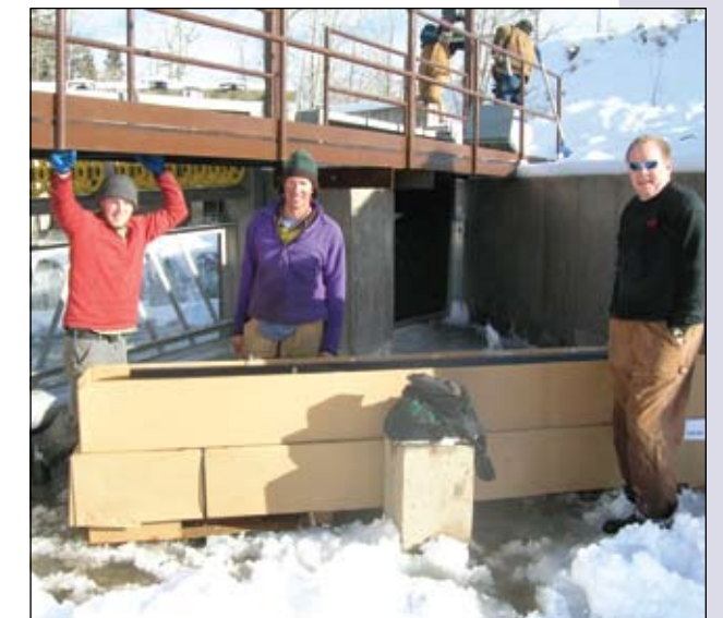
Paul Hood, Ned Cochran and James Reimer complete installation of the fish screen on Hog Canal, South Leigh Creek.
